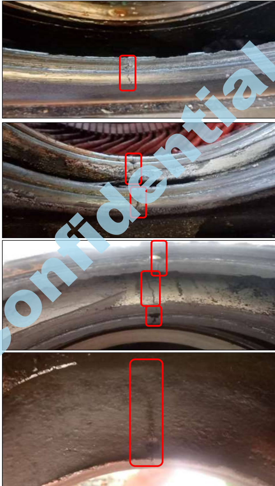
Fig 13, 14 & 15 & 16: Lower part bearing housing was found badly melted collar with internal deep long crack lines.
