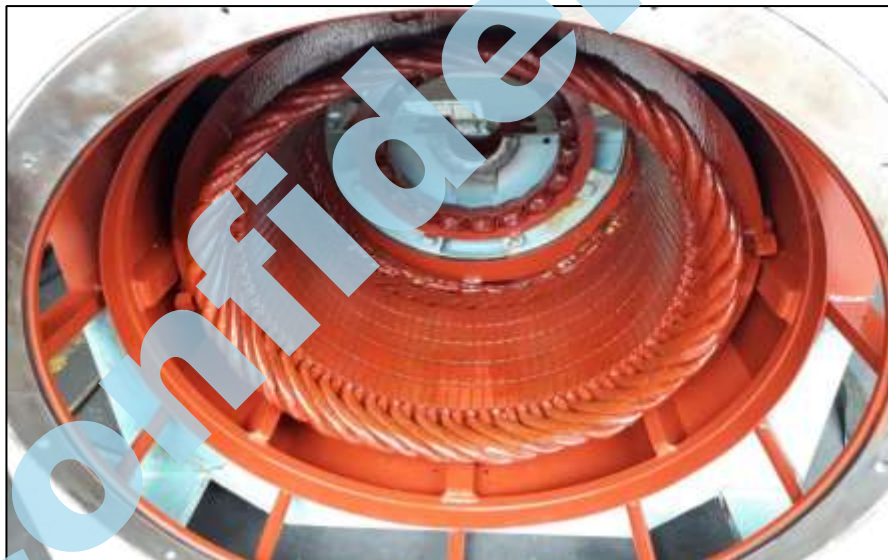
Fig. 17 & 18: Condition of Main Stator after servicing.
