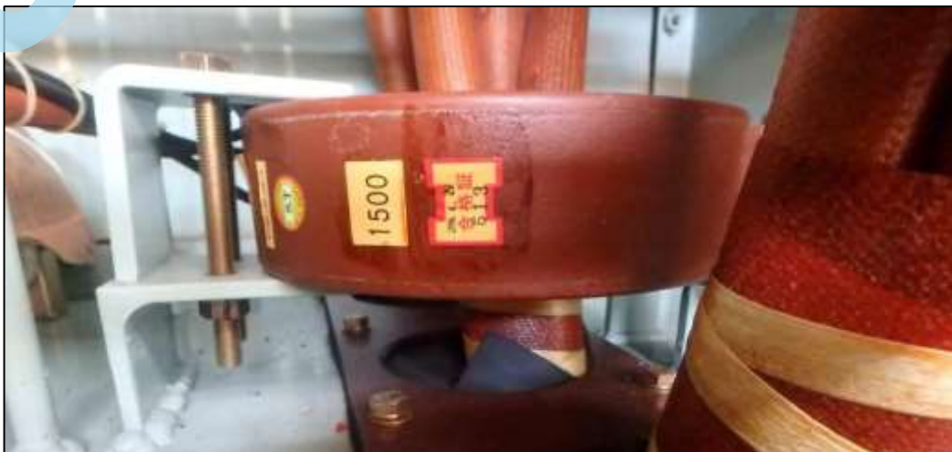
Fig. 28 & 29: Outgoing power supply terminals, some control terminals, CT & resistor after re-installed as per original.
