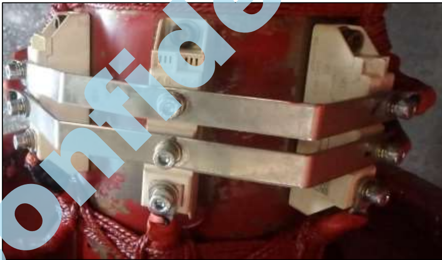
Fig. 24: Condition of Rectifier bridge diodes after renewed and installed as per original.
